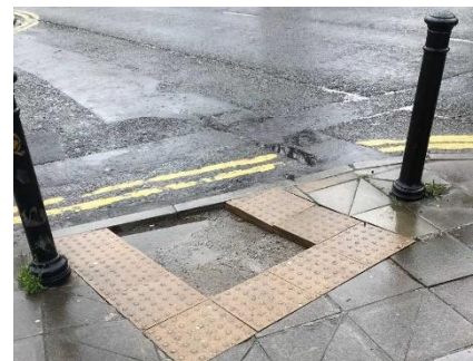
Figure 82: Unfinished tactile paving
