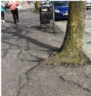
Figure 83: Tree roots creating uneven paving
