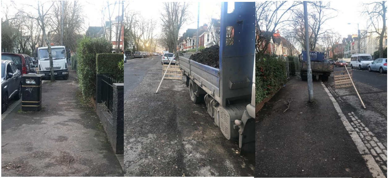
Figure 108: Road works and street clutter, Wellington Avenue
