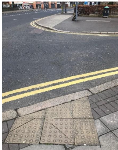
Figure 130: Cracked and missing tactile paving, Belfast
