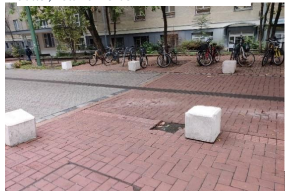
Figure 118: Crack and missing paving, Szeged Hungary
